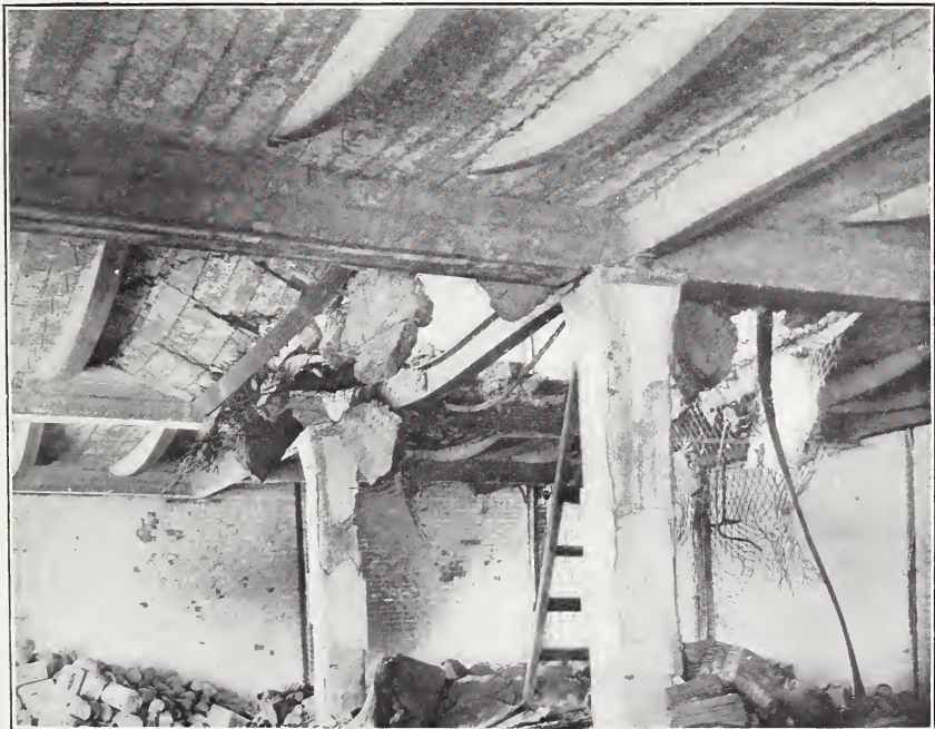
B. COLLAPSE OF FLOOR PANEL, CAUSED BY LOAD FALLING FROM A FLOOR ABOVE, THIRD FLOOR OF ÆTNA BUILDING, SAN FRANCISCO.
